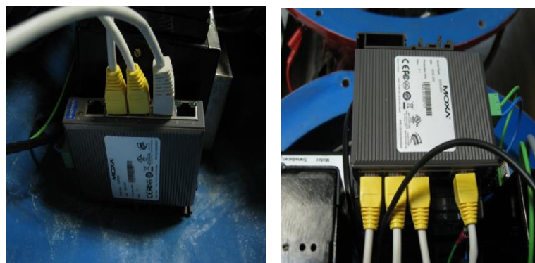
Figure 8. The switches inside the head and body of the Aegir Submarine
